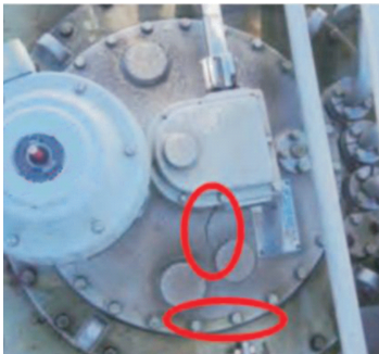
图 2 电弧故障导致 OLTC 结构破裂形貌图 [21] Fig. 2 Topography of rupture of the structure in arc fault OLTC [21]
